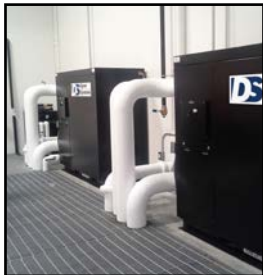
Coolant Storage and Distribution
