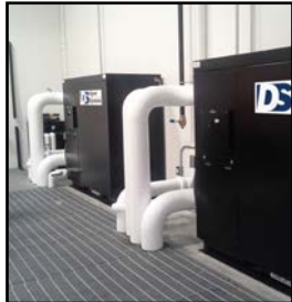
Coolant Storage and Distribution
