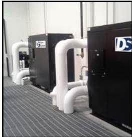
Coolant Storage and Distribution
