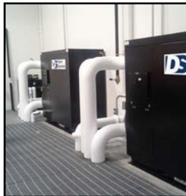
Coolant Storage and Distribution
