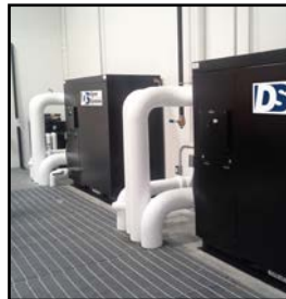
Coolant Storage and Distribution
