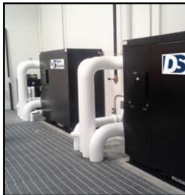
Coolant Storage and Distribution
