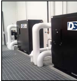
Coolant Storage and Distribution
