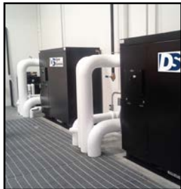
Coolant Storage and Distribution
