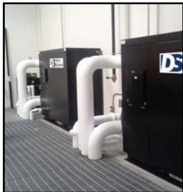
Coolant Storage and Distribution
