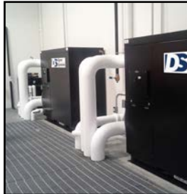
Coolant Storage and Distribution
