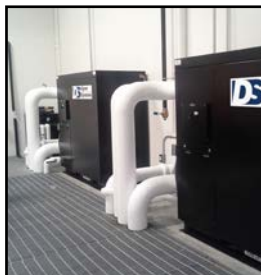
Coolant Storage and Distribution
