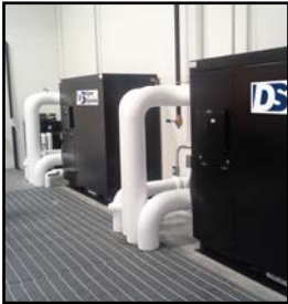
Coolant Storage and Distribution
