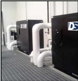
Coolant Storage and Distribution
