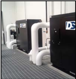
Coolant Storage and Distribution
