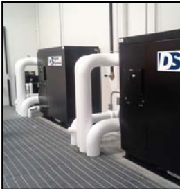
Coolant Storage and Distribution
