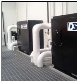
Coolant Storage and Distribution
