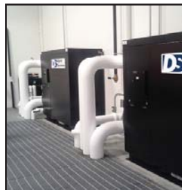
Coolant Storage and Distribution
