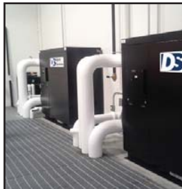
Coolant Storage and Distribution
