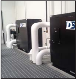
Coolant Storage and Distribution
