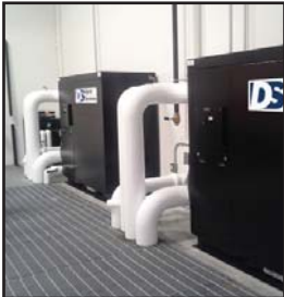
Coolant Storage and Distribution
