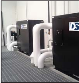
Coolant Storage and Distribution
