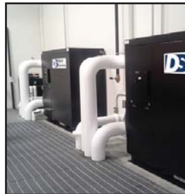
Coolant Storage and Distribution
