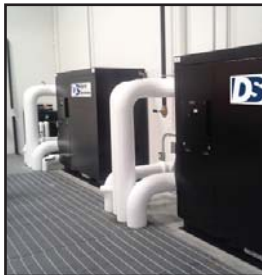
Coolant Storage and Distribution
