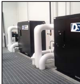
Coolant Storage and Distribution
