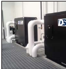
Coolant Storage and Distribution
