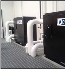
Coolant Storage and Distribution
