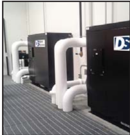
Coolant Storage and Distribution
